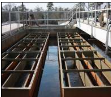
Fig 1: A typical coagulation tank in a drinking water treatment facility.
